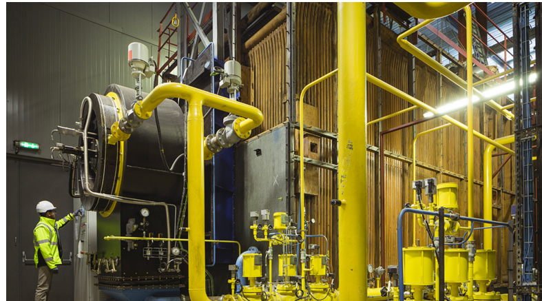
Thermal power plant
